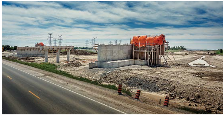
OPUCN relocated poles and other infrastructure to make way for development of the Highway 407 ETR, including the construction of an overpass where Simcoe St. will eventually cross the highway.
