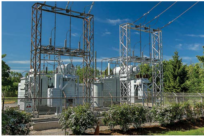
In 2013, OPUCN refurbished its Wilson Rd. substation (MS13), the company's fifth major substation upgrade.
